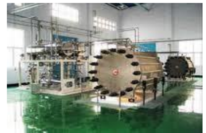
Water Electrolysis Equipment
