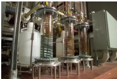
Water Electrolysis Equipment
